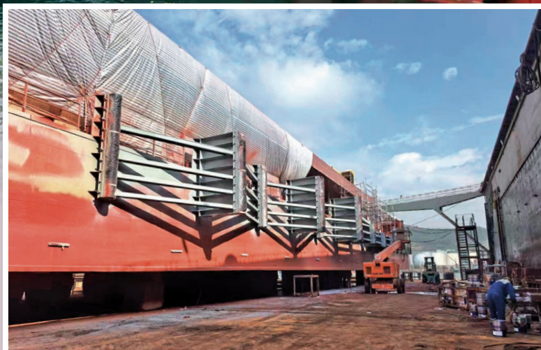
Berth No. 5 has been modified with an extended platform to accommodate extra-low freeboard ferries, enhancing operational resilience. 五號泊位經改建後增設延伸平台，以配合超低乾舷快船停靠，從而提升營運應變能力。
